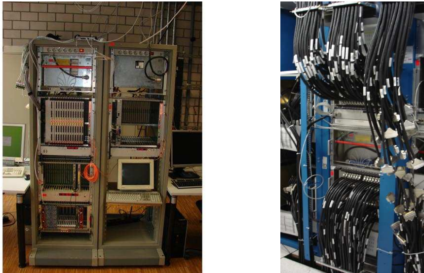
Figure 2.6: The full-crate test set-up built in the ATLAS Lab@KIP to test the PPMs (a) and details of the installation of the PPr System at CERN, in the electronics cavern of the experiment - as of August 2007 (b).
