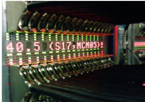
Figure 2.10: Detail of a fully equipped Pre-Processor Crate
