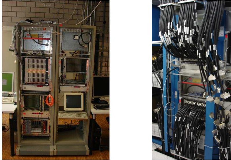
Figure 2.6: The full-crate test set-up built in the ATLAS Lab@KIP to test the PPMs (a) and details of the installation of the PPr System at CERN, in the electronics cavern of the experiment - as of August 2007 (b).
